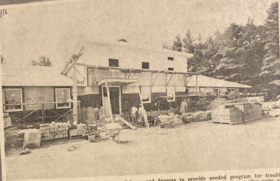
NEARING COMPLETION in Allenstown is first Salvation of Youth cottage in Somaschan Fathers' non-sectarian, pilot-project for prevention of juvenile delinquency. Called Pine Haven, cottage gives tangible evidence of concern of civic-minded citizens who contributed both effort
